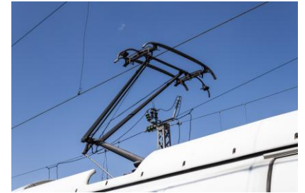
Contact between catenary and pantograph
